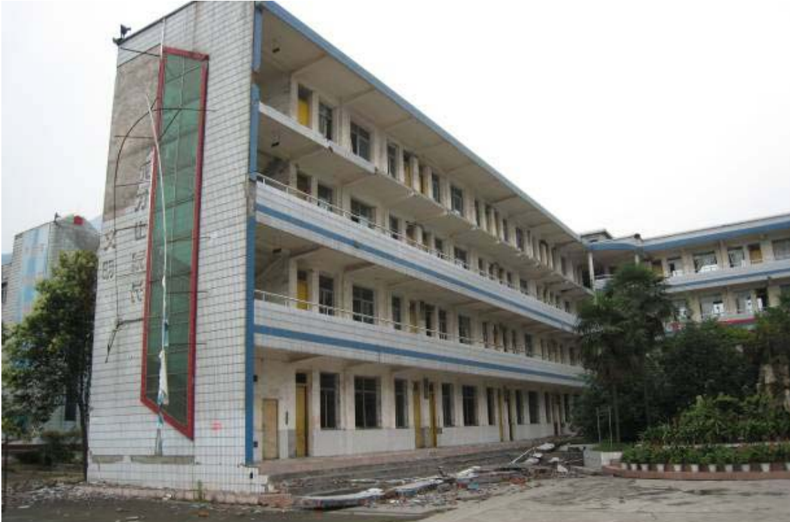
Photo 3: Hanwang middle school in Mianzhu City, VIII MMI scale, with slight damage. Two students were killed because of the collapse of brick parapet in 3 rd storey
