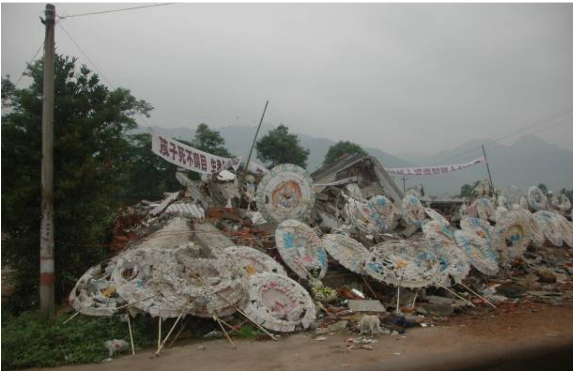
Photo 4: Jiulong elementary school, Jiulong Town, Mianzhu City. Among 200 students only 30 could survived. This photo shows only the mourning signs (made of white paper) placed above the collapsed building.
