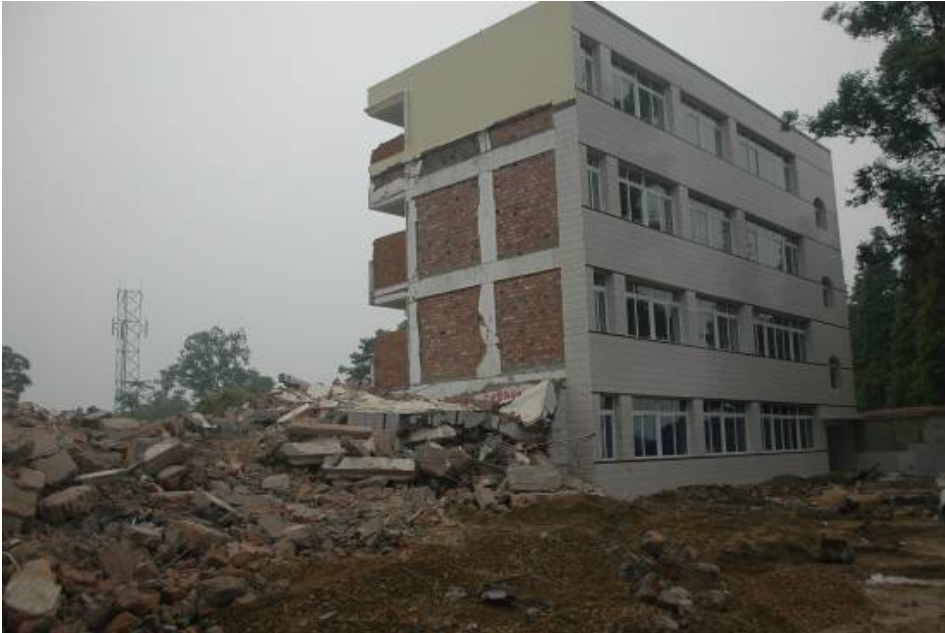
Photo 1: A school building in Shifang City. The intensity at this place was about 7.5 MMI. The right side building is a reinforced concrete structure built in 2005 and it had minor damaged. The left school building was brick masonry with ring beams, columns and prefabricated slabs as floor built in 2000. It was heavily damaged, but did not collapse and no students were injured. The left side school building was dismantled later.
