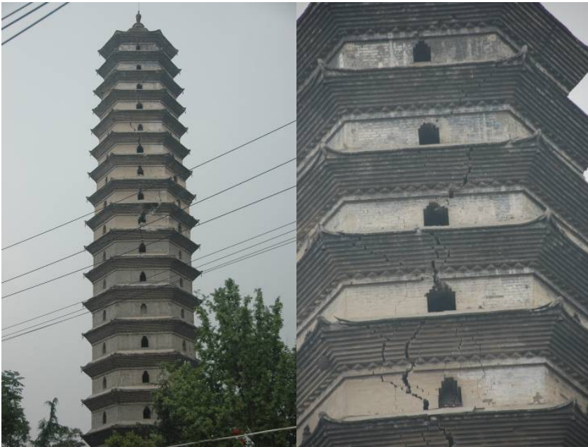
Photo 6: Tall brick tower, built during Ming Dynasty, about five hundred years ago, in the Dujiangyan City. The intensity was VIII MMI and it was moderately damaged in the upper part. Compared with present building, the masonry quality is considerably fine.
