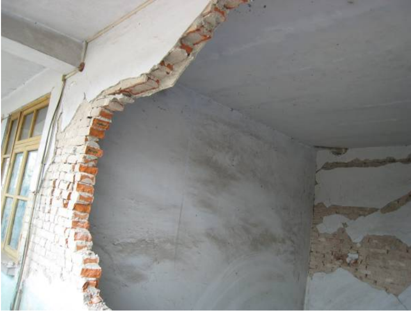
Photo 5: 3-storey brick building, heavily damaged during the Earthquake. The intensity was about 7.5 MMI. The quality of masonry construction was not good: (1) the strength of mortar was not sufficient, and it could be cracked by hand; (2) the joints were not staggered.
