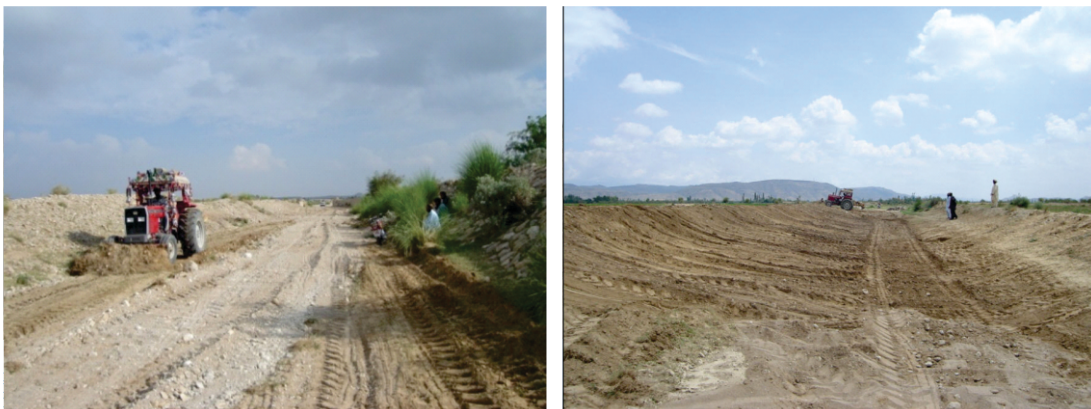
Fig. 2. De-silting, aligning, grading and compaction work at experimental site at Rarkan, Baluchistan.
